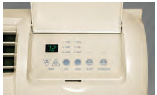
Temperature control panel
